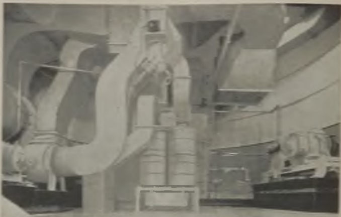
Ventilation plant is installed at the base of one of the main shafts
