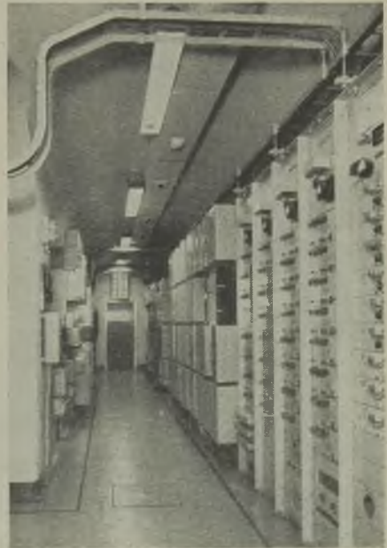
Original exit passage from the lifts to the station platforms now serving as an apparatus gallery
