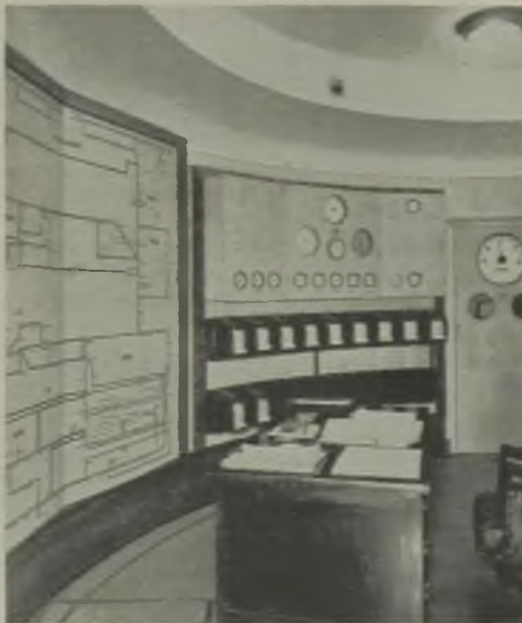
The equipment in the national control room is mainly in the form of a complete grid diagram setting out the various area schemes and inter-connecting tie lines
