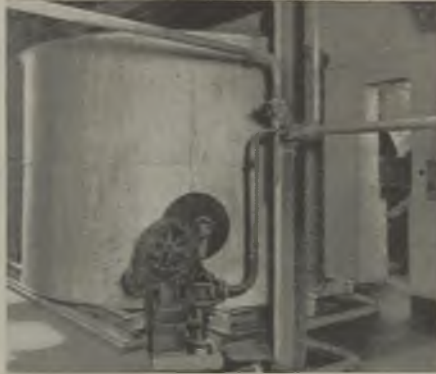
Thickener tank with pump, at Dalehall Mills
