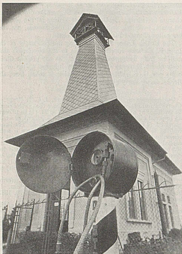
COMPRESSED METHANE GAS FILLING STATION, ITALY 4500 pounds per square inch
