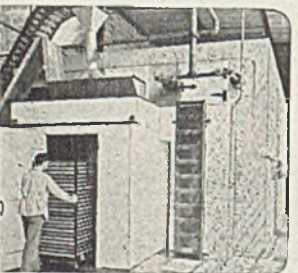
Frick-Freezer Tunnel operated at -35° F. at Lancaster, Pennsylvania.
