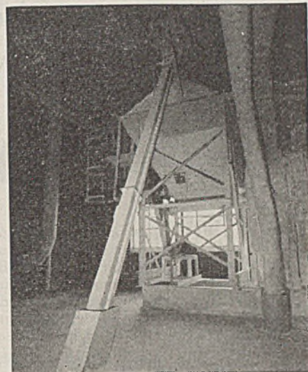
Discharge end of Bulk-Flo, which discharges into storage hopper, which in turn discharges into dryer.
