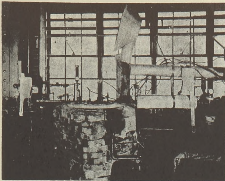
Figure 3. Pyrolysis Furnace in Butadiene Pilot Plant, Showing Pre-heater, Gas Heating System, Spray-Quench System, and Butadiene Stripping Column
