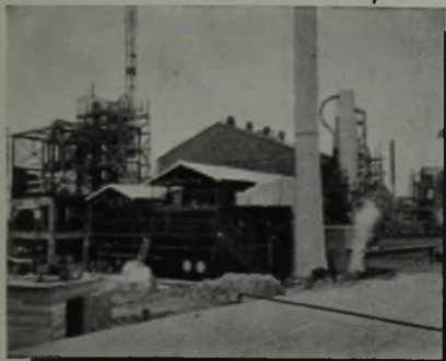
This 4400 barrel per day Benzol-Ketone Dewaxing Plant was completed in exactly twenty weeks from date of contract.
