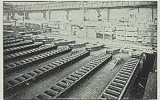
A typical Standard Conveyor installation in one of the country's largest steel plants.
