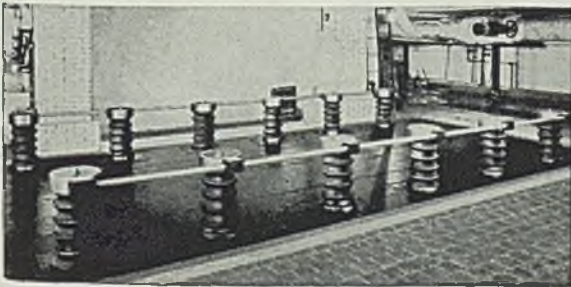
Spring bases in position ready for forming of floating slab upon which the engine is mounted.
