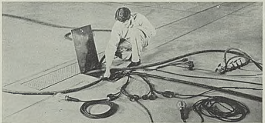
Electrical, compressed air and other connections are obtained through access openings spaced at regular intervals throughout the plant. When not in use these openings are covered with cast iron floor plates
