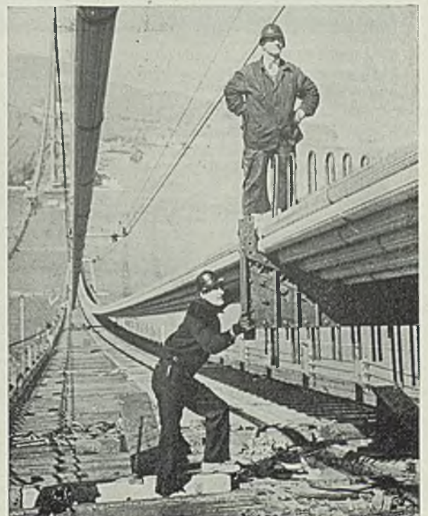
This view of the Golden Gate bridge across the entrance to San Francisco bay looks north toward the Marin hills. In the foreground workmen are placing ricket frames in position. The foot bridge is 18 feet wide and nearly 8000 feet long
