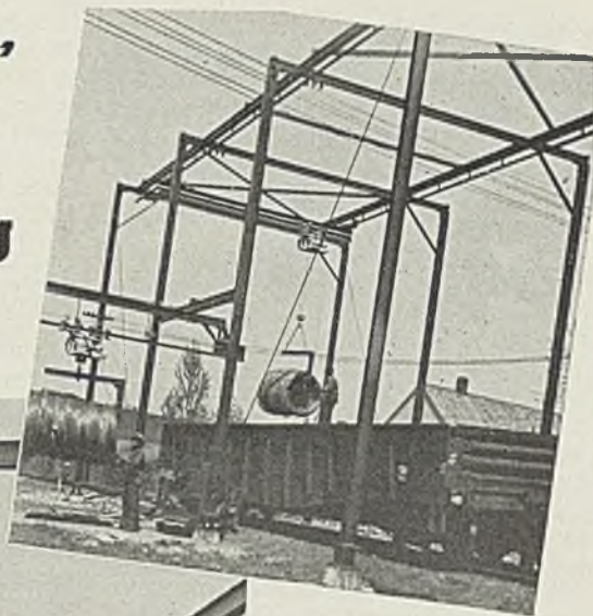
Two men unload car of rod in 1½ hours with crane and electric hoist.
