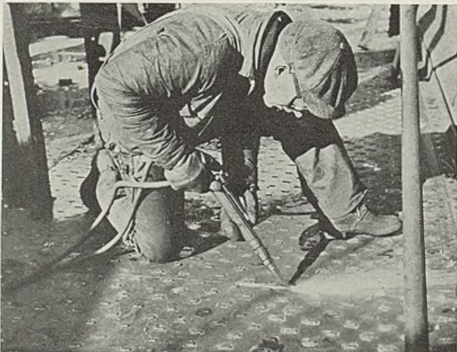
Fig. 11—Manual application of full-U grooving on deck plates of a dredge. Groove is being made between two plates butted together and welded underneath to form a shelf
