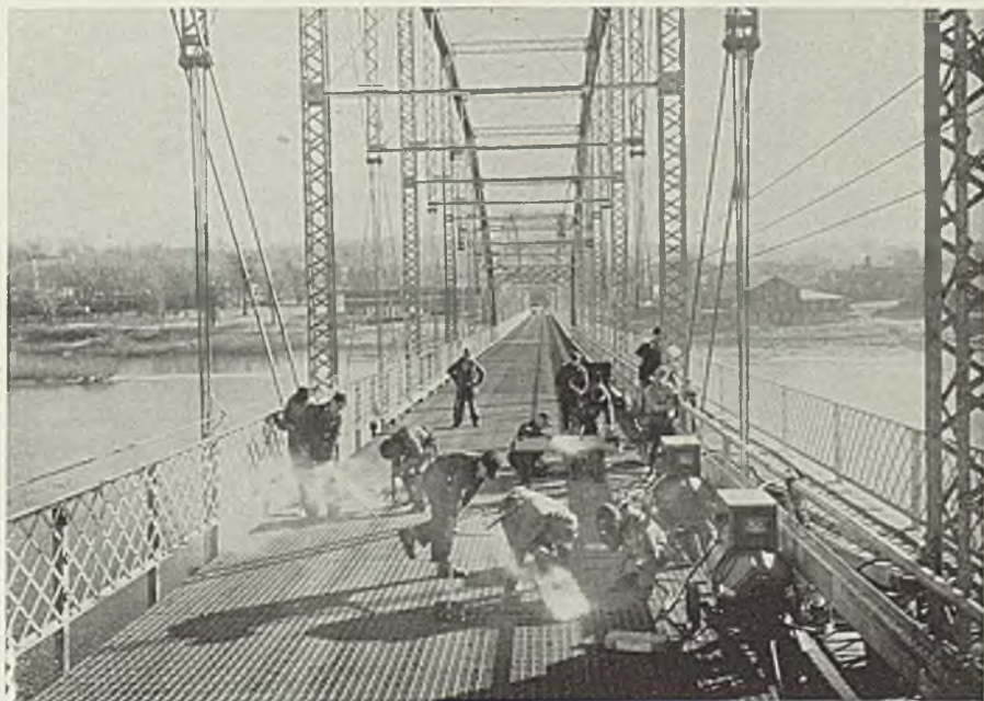
■ Steel grating welded to the stringers replaces wood flooring formerly used on this bridge over the Mississippi river at Clinton, Iowa. By laying the grating in sections, Lyons & Fulton Bridge Co. is replacing the deck without disrupting traffic. Photo courtesy General Electric Co., Schenectady, N. Y.
