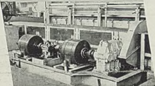
Jones Herringbone Reducers operating furnace in steel mill. Drive consists of two motors with single type and double type reducers coupled in series in order to obtain two widely varying speeds.
