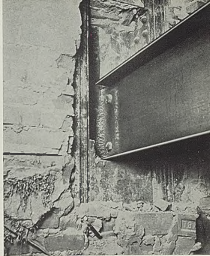
Fig. 13—Arc-welded connection of beam to an existing column . . . easily and quickly made
