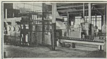
AIRPLANE PROPELLER BLADES and other aircraft parts are securely joined in this E.F. copper brazing furnace—one of a number of types of continuous and batch type installations made by The Electric Furnace Co., Salem, Ohio for copper and brass brazing and silver soldering, large and small assemblies.
