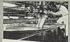
Tanks lined with IngAclad SHEETS protect color and flavor of Corn Syrup.
