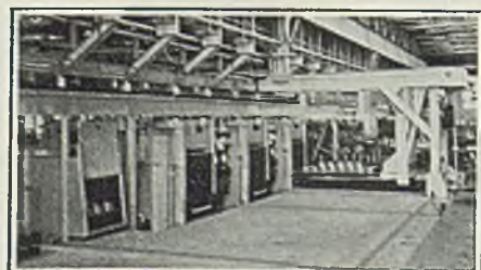
BRASS FOR CARTRIDGES and other products are uniformly treated in various types of EF continuous, semi-continuous and batch type furnaces. The above installation shows 3 gas fired, hearth type forced circulation furnaces with quench, cooling chamber and handling crane—one of several similar installations made in prominent nonferrous plants by The Electric Furnace Co., Salem, Ohio.
