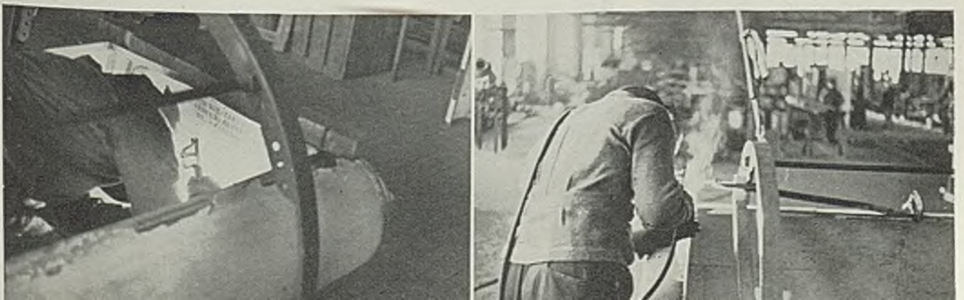
Fig. 7—Next, outside tack welds are ground off and outside bead deposited as shown here at right below
