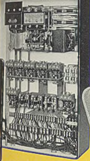
A-B custom-built control panel for a 24-spindle, 3-station drilling machine.
