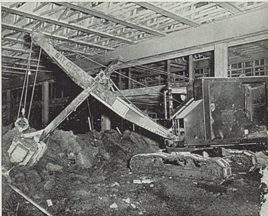
■ New defense plants are being erected with such speed that buildings are well along toward completion before excavation for floors has been started. Here is a case in point, inside the Ford aircraft engine plant in Detroit.
