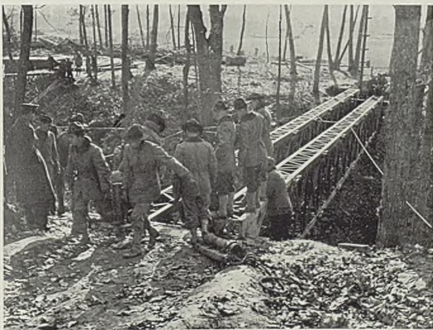
■ Portable, experimental steel girder bridges, often with five center and two end sections, for throwing over small rivers, are being constructed for the army engineers' corps, Ft. Belvoir, Va. The sections are equipped with wheels at ends for mobility. These bridges are more elaborate than one-piece ramps for spanning ditches. Photo, U. S. Army Signal Corps
