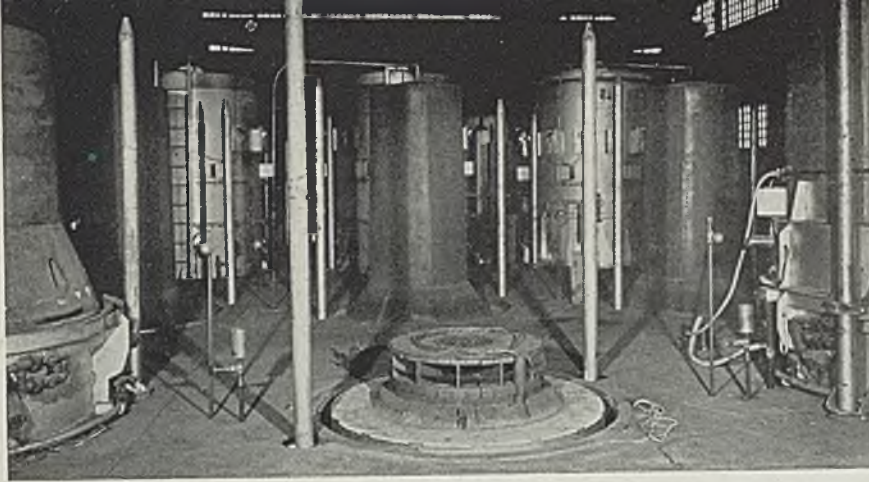
Fig. 2—General view in annealing department at plant of Superior Steel Corp.
