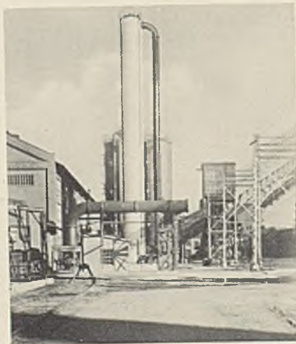
The usual wood hurdles are replaced in this new scrubber with steel spiral packing and this one scrubber has the same recovery efficiency as customarily obtained with two scrubbers in series.
