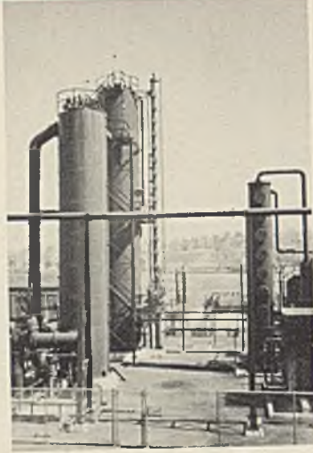
Here is a simple light oil recovery system at a gas plant with a capacity of 6,000 gallons of crude light oil per day. It has no rectifier but has a continuous motor benzol recovery column. The scrubber is a single steel spiral-packed tower.
