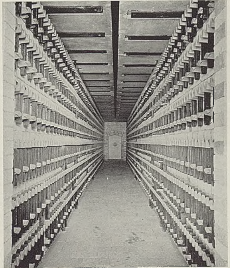
Fig. 2—Continuous electric enameling furnace, 1200 kilowatts rating, interior view of outgoing side. Heating elements are divided into 12 sections; 52 thermocouple locations are provided
