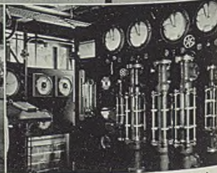
STILLS for chemicals are precision-operated from control rooms by Foxboro Temperature, Flow and Potentiometer Controllers.
