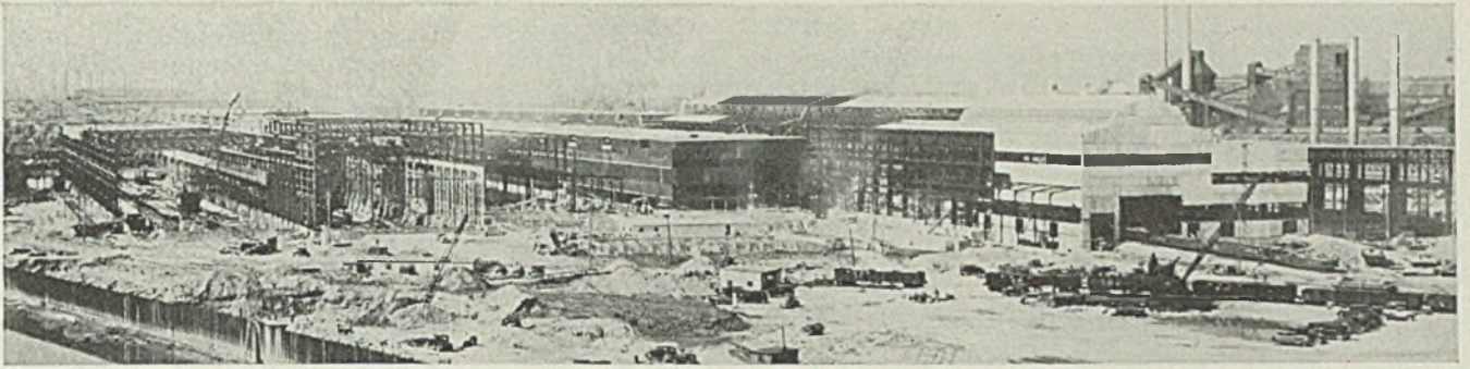
Republic Steel Corp.'s new 98-inch continuous strip mills in the Cuyahoga valley, Cleveland. The cold mill buildings are seen at the left. The hot mill group, to the right, is already under roof and partially enclosed
