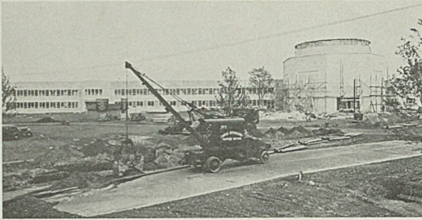
Now nearing completion in the New York World's fair group is the administration building. Several hundred tons of steel were used in its construction
