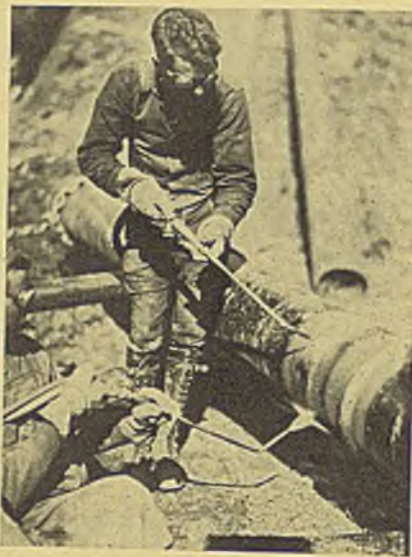
Wrinkle bending is one of many localized heating applications easily done with an oxyacetylene torch
