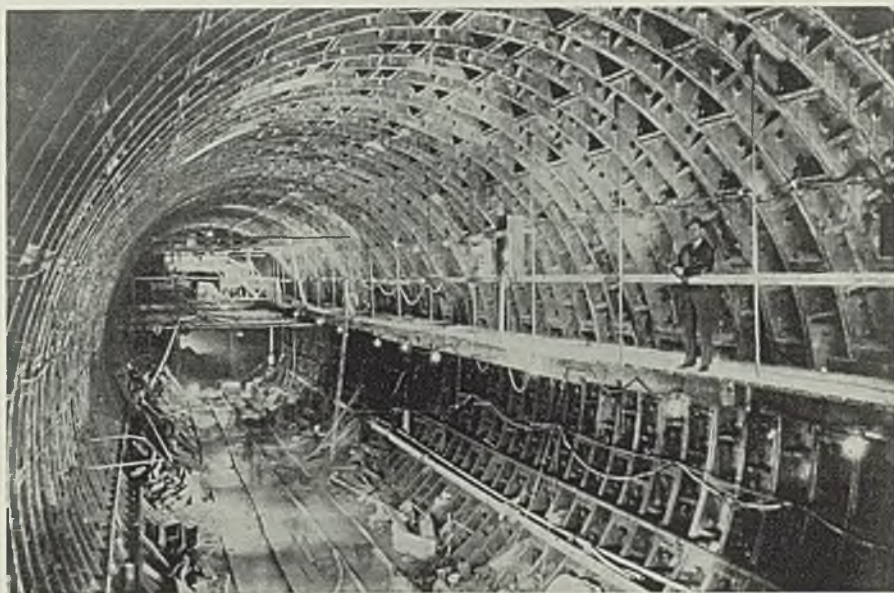
■ Cast iron rings 30 feet in diameter and weighing 3200 pounds each form the lining for Queens Midtown tunnel under East river, New York. To make tunnel waterproof, grooves between rings were caulked with lead. Rings were prepared for caulking by power-driven wirewheel brushes to clean off rust and a wax coating. Photo, courtesy Osborn Mfg. Co., Cleveland
