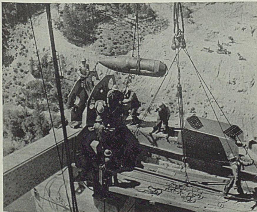
■ Much as it may look like one, this is not a shell: it is a forged steel pin which will help hold together two spans of the Pit river bridge being built over an arm of the Shasta reservoir in California. Pin is 22 inches in diameter and 8 feet long. NEA photo from Bureau of Reclamation
