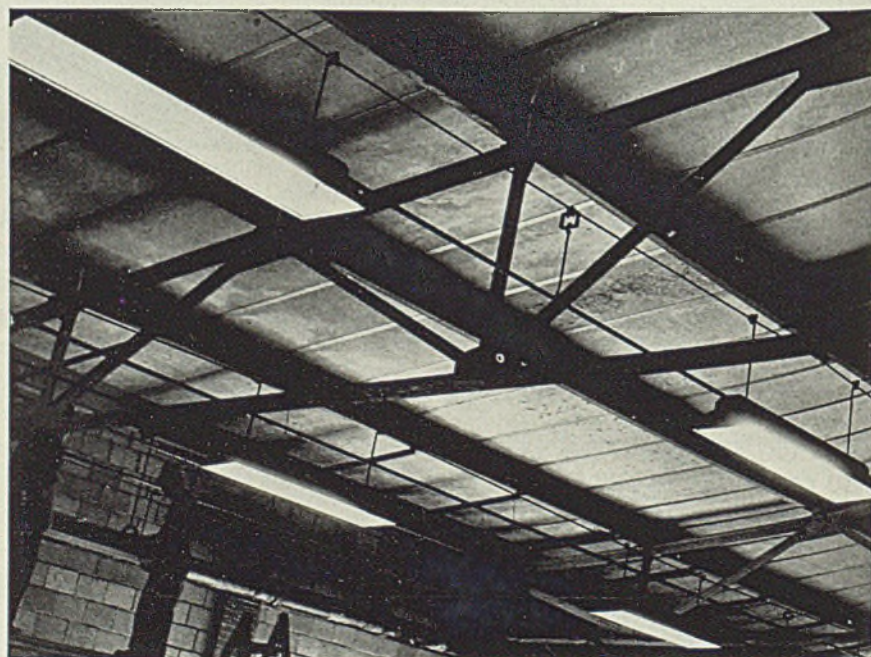
■ Method of supporting the roof by means of bridge-type prefabricated steel trusses is apparent in this picture, which also shows how fluorescent luminaires are supported from cables
