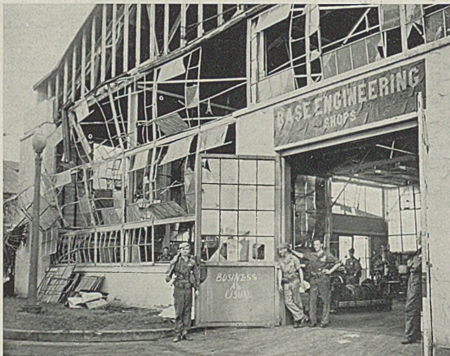
■ HONOLULU, T. H.: Although not struck by a bomb, a repair shop at the airport here was wrecked as shown by this picture when a missile exploded nearby. Next day the garagemen chalked "Business as Usual" on the doors. NEA photo
