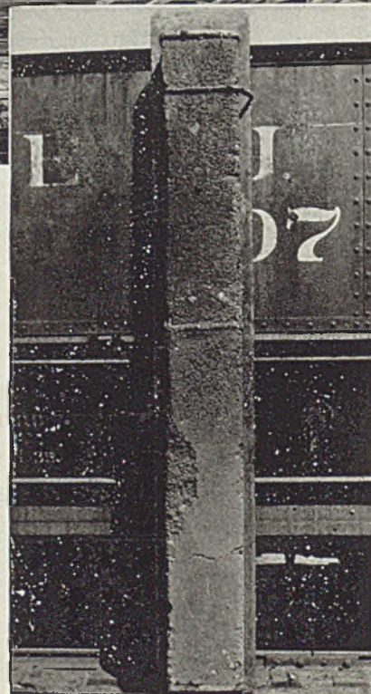
• Important coke-plant use of LUMNITE — Refractory Concrete Door Lining. This picture shows a Refractory Concrete Lining after more than 5 years' continuous service.
