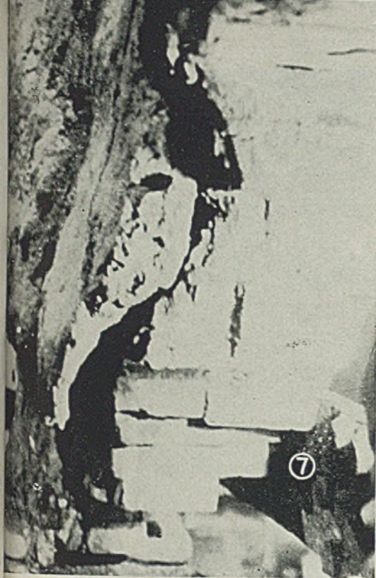
Fig. 7—Cross section of bosh wall, with coolers removed. Temperature contours in brickwork are apparent. Attacked zone is thicker midway between coolers than in immediate vicinity of coolers
