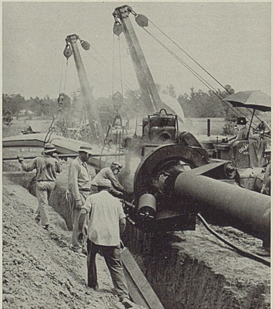
Protective coating of tar-like substance is applied to 24-inch pipeline which will carry crude and heating oils from Texas to the East coast. An asbestos-paper covering will complete the coating. NEA photo
