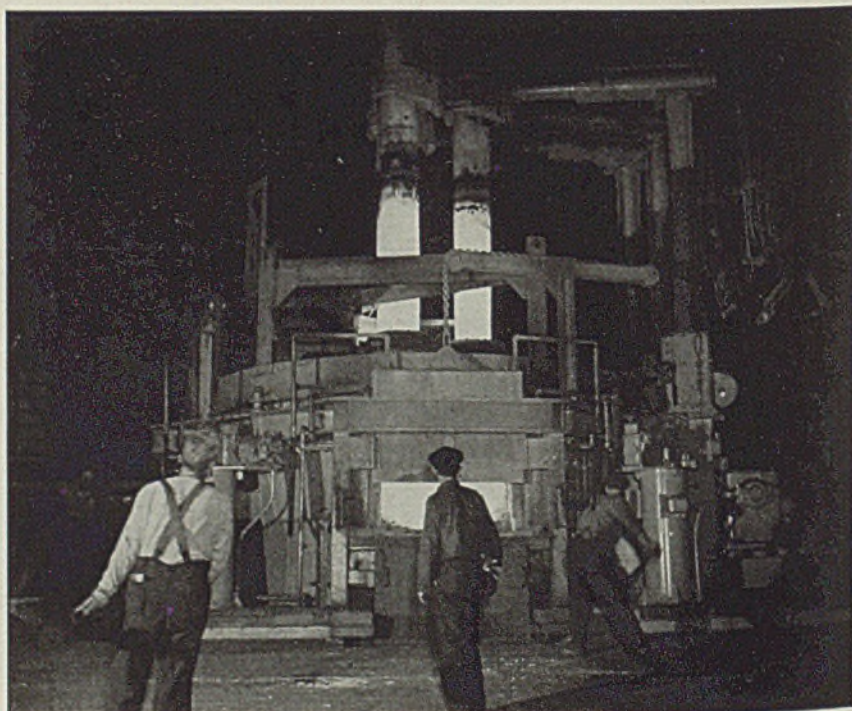
ELECTRODES of the first of three new electric furnaces of Carnegie-Illinois Steel Corp.'s Monongahela Valley expansion about to be lowered into position. The new furnace will produce vitally needed war steels (STEEL, Nov. 30, p. 45)
