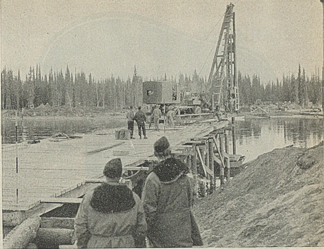
This temporary bridge on the upper Liard River will be replaced by a steel span.
