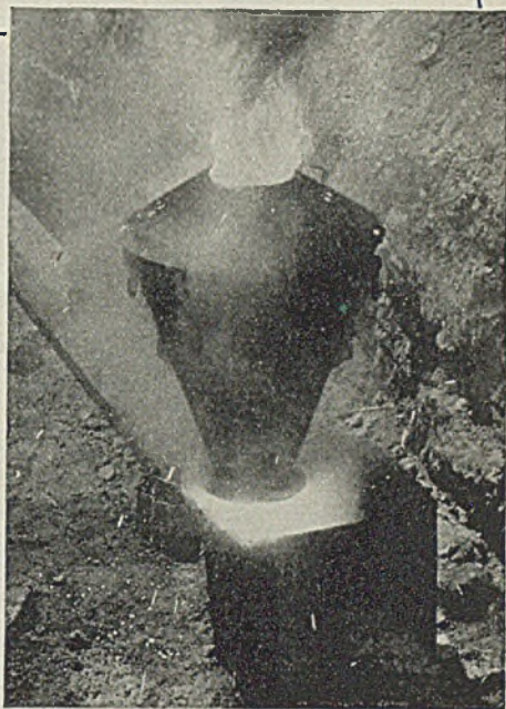
Pouring the molten Thermanit. A five-man crew completed six Thermanit welds daily.
