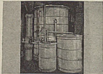
MILK PROCESS PLANT Single-tank ILLCO Combination-Regeneration Boiler Feed Unit, regenerated simultaneously with salt and acid; produces same results as Duplex Equipment above. Cypress tanks avoid use of critical materials.
