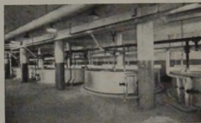
Thirteen tons of 3/16" IngAclad Plate used for top section and covers of these Soap Kettles installed in a Canadian plant.
