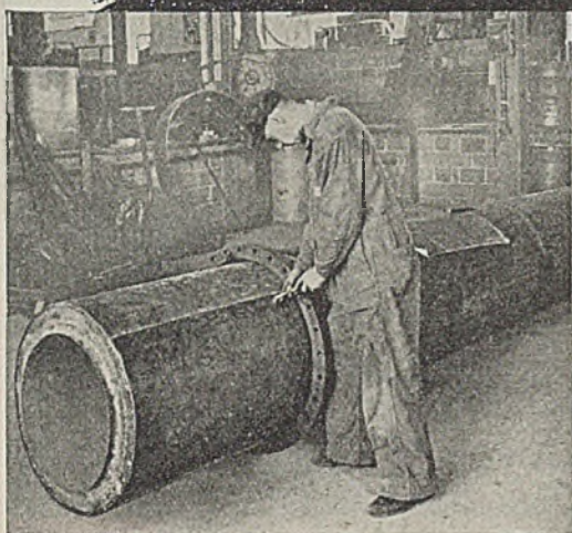
Insidline installations in pipe from 2" I. D. to 36" I. D. are made with a cartridge type of insulation that is built up first and then drawn into the pipe.
