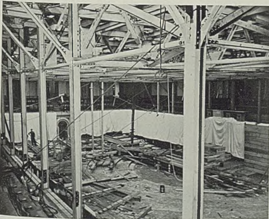
■ Temporary steel girders support the ceiling of the house of representatives, Washington, while workmen prepare to reinforce the roof, which has been declared unsafe. Acme photo
