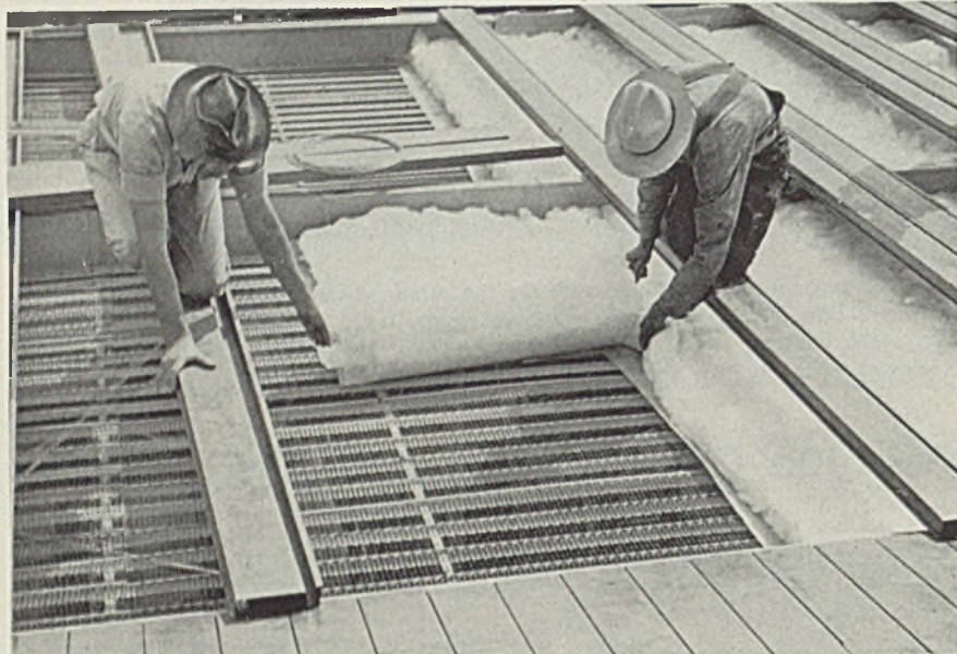
■ White glass wool will blanket roofs and walls at bomber assembly plants. Runner channels, which are welded to steel purlins, 33 inches on centers, support the \frac{3}{8} -inch ribbed expanded metal lath on which is spread a thin light reflecting mat of fibreglas, and a 3-inch blanket of white fibreglas for sound absorption and insulation. This in turn is covered by a metal deck, sections of which serve as temporary working platform. Fibreglas insulating board and several layers of special roofing materials are applied over this. Construction of side walls is similar, except that outer covering consists of ribbed steel sheets, painted
