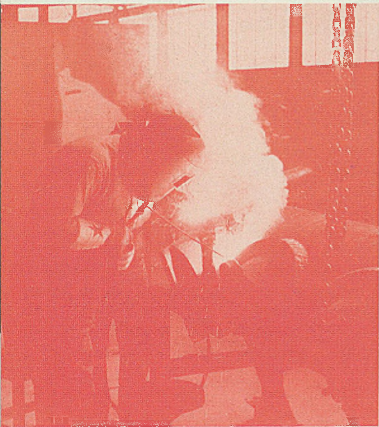
Fig. 1—For many fabrications such as power plant piping it is worth while to have chart records of the actual welding. Here records are being taken while welding headers
