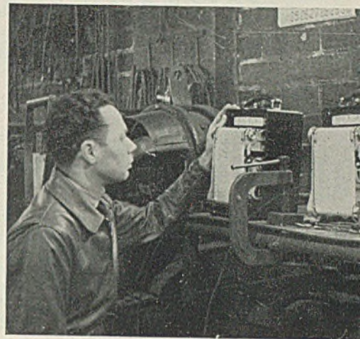
Fig. 4—A typical plant installation of graphic recorders for the purpose of production control of welding operations. All illustrations furnished by Esterline-Angus Co. Inc., Indianapolis, Ind.
