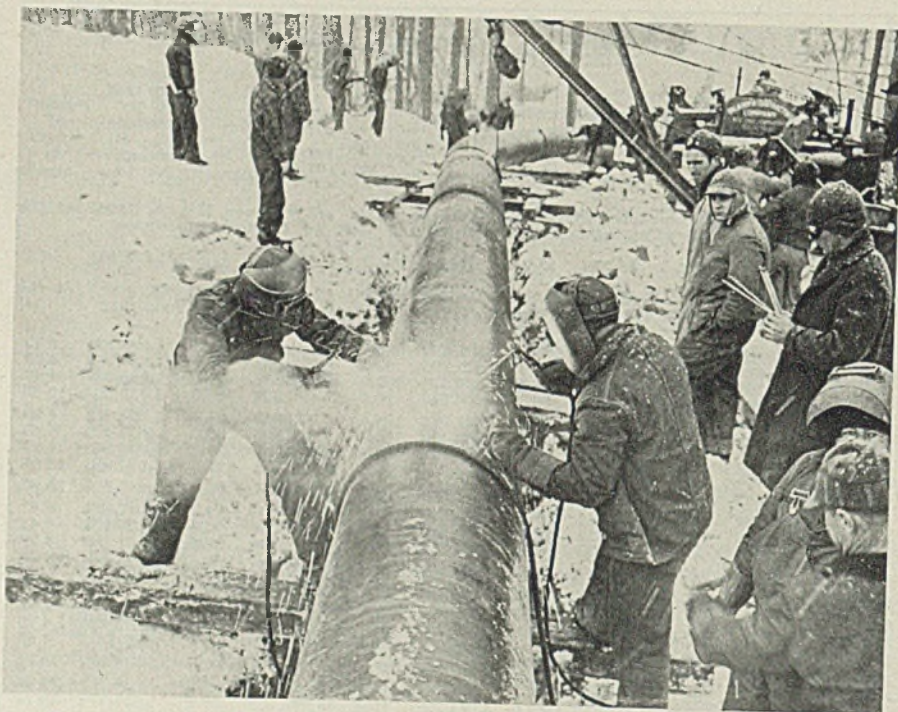
BAD weather doesn't delay laying of the "Big Inch" pipeline from Texas to the eastern seaboard. Above, welders tack the sections together in the Pennsylvania hill country. Shaped to conform to the contour of the countryside, the huge pipe rests on skids while being assembled. Shipments for the start of the line in Texas were begun last July. NEA photo
