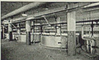
Thirteen tons of 3/16" IngAclad Plate used for top section and covers of these Soap Kettles installed in a Canadian plant.
