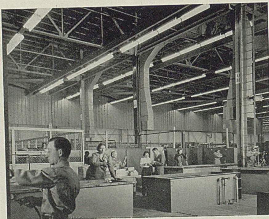
Ventilating ducts are provided in the cadmium plating section. Metal curtains extending 10 to 15 feet below the bottom chord of the trusses trap, process heat and gases exhausted directly to the outside through fans and blowers. Photos by courtesy of Austin Co.
