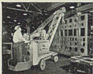
In erection of control panels, Baker relieves overhead cranes for other work.
