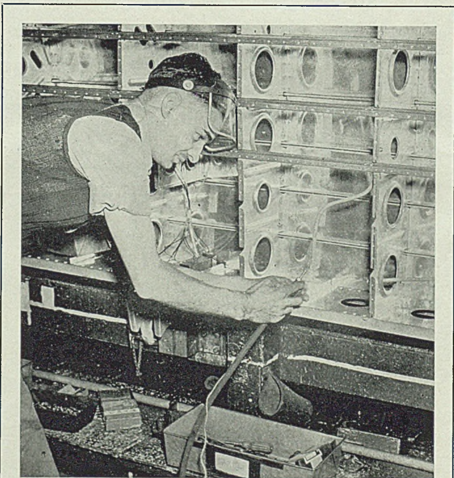
TIME SAVER: Seventeen per cent saving in time has been effected at the main aircraft plant of Fisher Body division with adoption of an employe's idea of blowing a piece of string through the conduit with the aid of an air hose, and then pulling the wire through after attaching it to the other end of the string. Former method was to push the wire through the conduits in horizontal stabilizers first, but this often proved troublesome because of the many bends in the conduit
