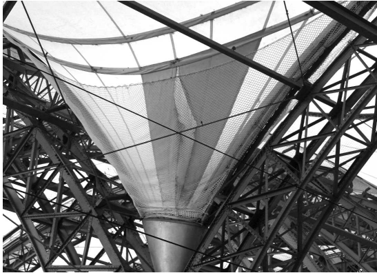
Fig. 4. One of the damages in the Dresden railway station roofing (author)
