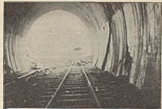
Abb. 33. Querrisse am Tunneleingang (Atami-Bahn).
