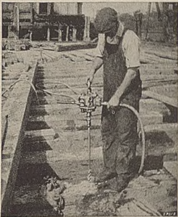
Fig. 25. —A four cylinder piston type wood borer drilling 1\frac{1}{2} in. holes in 12 x 12 timbers on bulkhead construction work.
